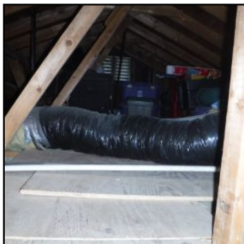
ATTIC AREA Duct Work
