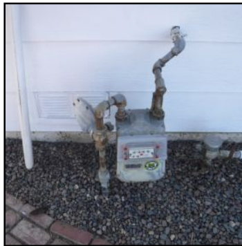
ELECTRICAL/GAS SERVICE Main Gas Valve
