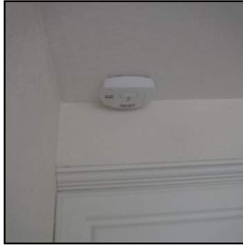
INTERIOR Carbon Monoxide Detectors
