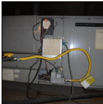
HEATING/AIR CONDITIONING Heaters
