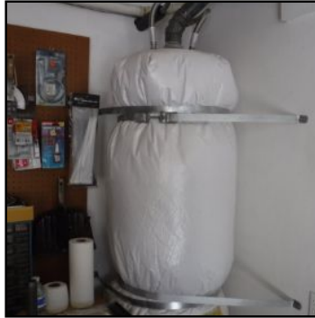
WATER HEATERS Water Heaters Condition
