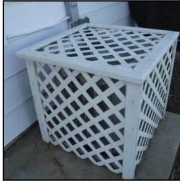
HEATING/AIR CONDITIONING Air Conditioning Compressors
