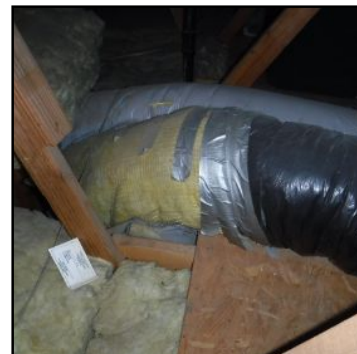
ATTIC AREA Duct Work
