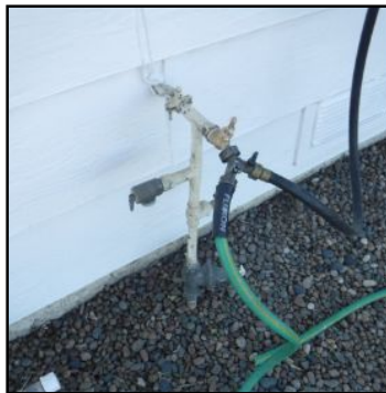
GROUNDS Main Water Valve
