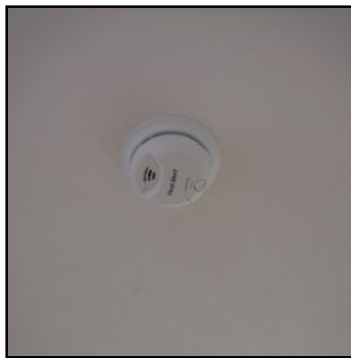
INTERIOR Smoke Detectors
