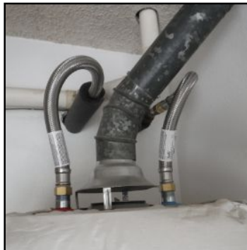
WATER HEATERS Plumbing
