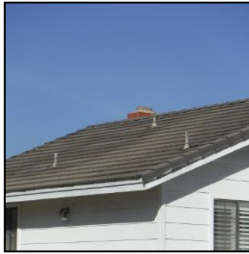
ROOF Vents and Vent Caps
