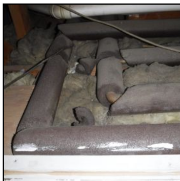
ATTIC AREA Plumbing
