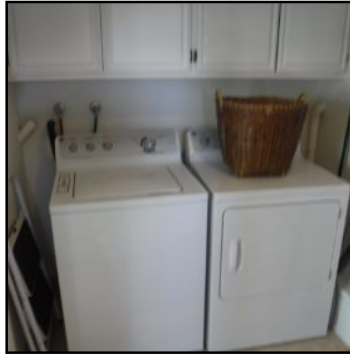
LAUNDRY AREA Wall Conditions
