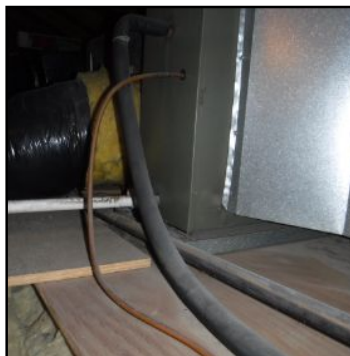
HEATING/AIR CONDITIONING Refrigerant Lines
