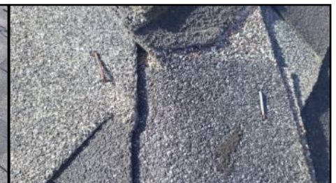
Exposed nails on roofing material - recommend sealing all fastener heads
