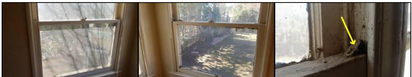
Stuck in position - needs to be serviced
