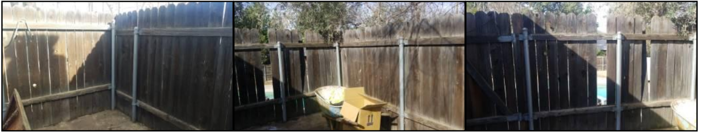
Damaged fencing/walls - needs to be serviced
