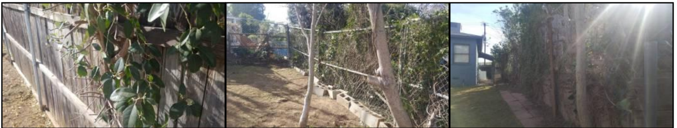
Vegetation or trees are affecting the fencing/walls in areas - needs to be serviced
