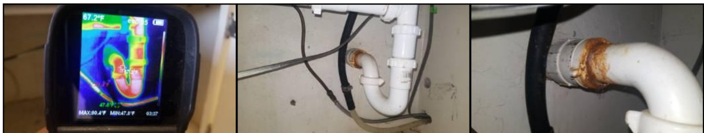
Corrosion is present at plumbing areas - this is a sign of slow leaking and should be serviced
