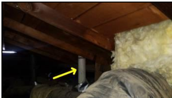
Masonry/cement/transite type vent pipe in the attic - needs to be serviced and possibly upgraded to newer style vents
