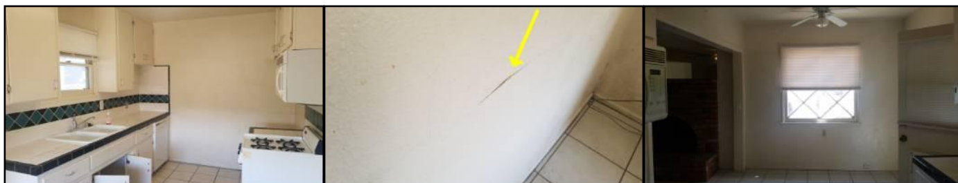
Large crack - recommend servicing
