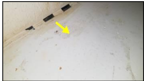
Visible leaking under sink - needs to be serviced
