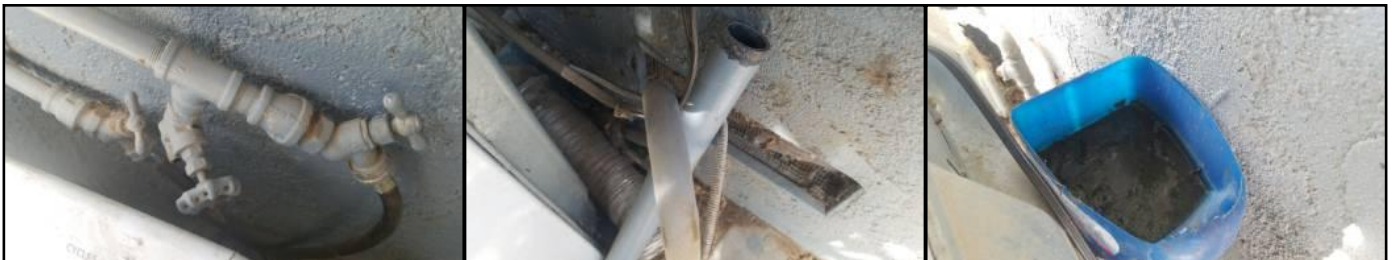
Drain trap is clogged - needs to be serviced
