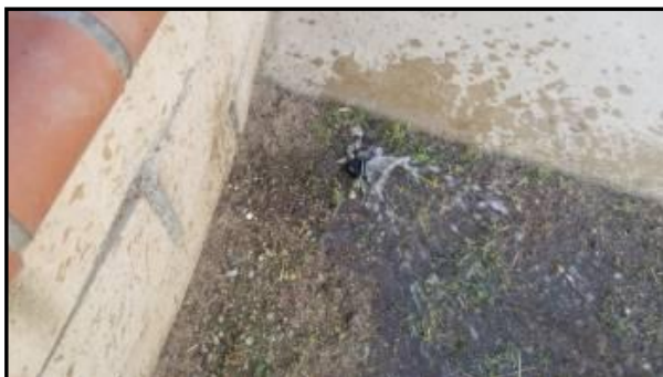
Low water flow at sprinkler heads - needs to be serviced
