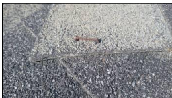
Exposed nails on roofing material - recommend sealing all fastener heads
