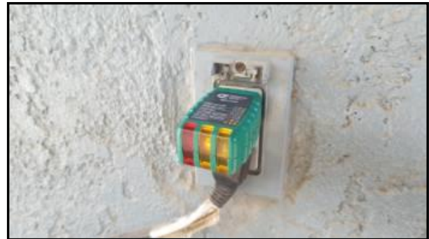
Missing exterior cover
