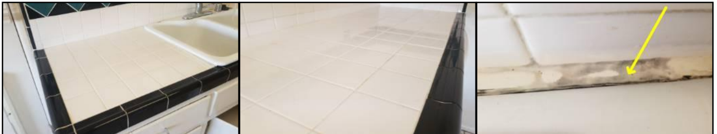
Gaps at countertop joints - needs to be serviced
