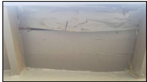
Deteriorated in areas - needs to be serviced - consult the termite report
