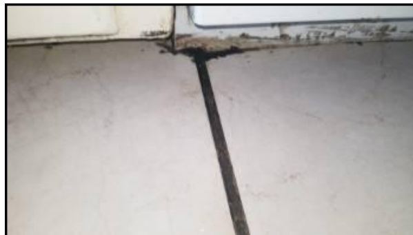
Leaking from the front door - needs to be serviced
