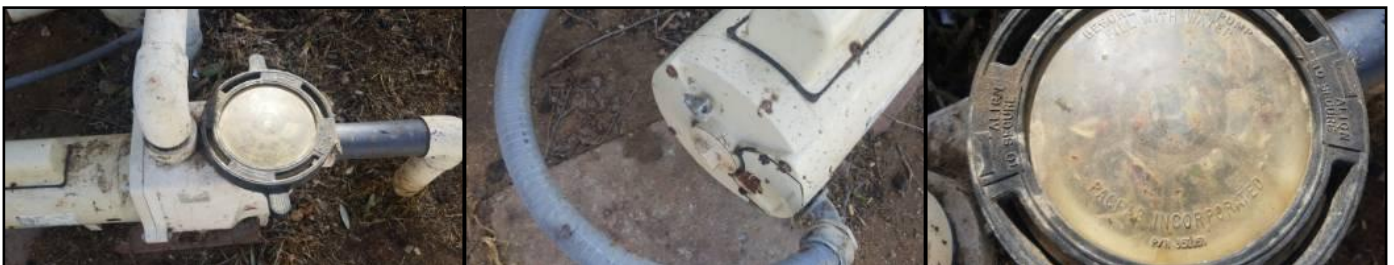
Missing bonding wire
