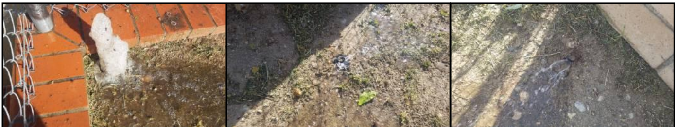
Missing sprinkler heads - needs to be serviced
