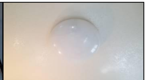
Some bulbs defective/missing/light(s) did not function - check bulbs/consult electrician to further evaluate
