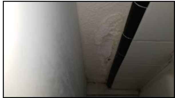
Damaged in areas - needs to be serviced
