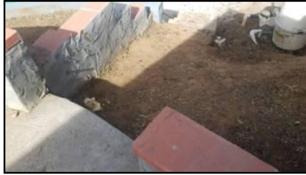
Missing steps - unsafe - needs to be serviced
