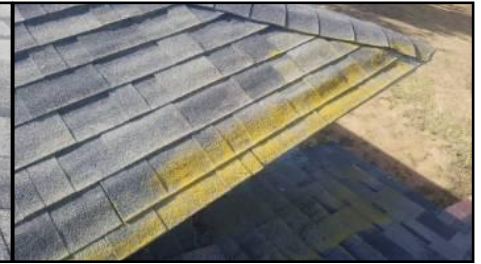
Sign of moisture accumulation and lack of sunlight for drying - recommend servicing as part of seasonal maintenance
