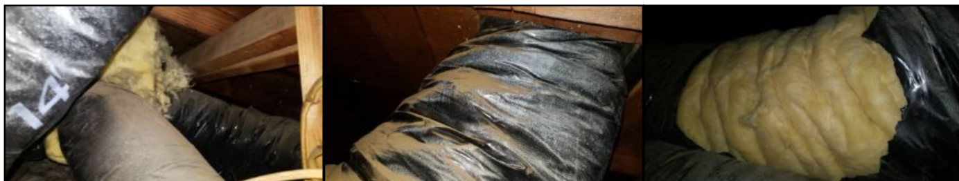
Outer wrap damaged - needs to be serviced
