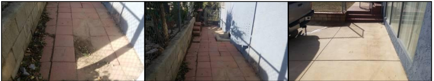
Walkway displacement/uplifted/uneven areas - potential trip hazard - needs to be serviced
