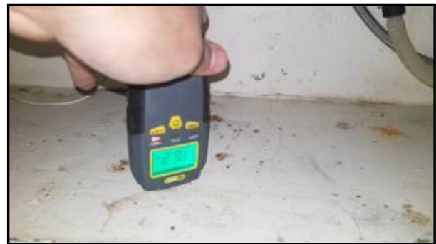
Stained/blistered area(s) - moisture present at time of inspection - needs to be serviced/further evaluated
