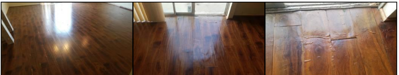
Wood flooring is swollen/cupping/lifting - evidence of a past moisture problem - needs to be serviced
