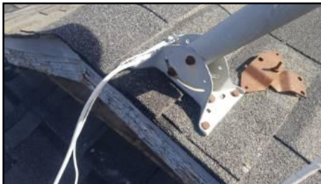
Satellite dish fastened direct to roof - screws will need periodic caulk maintenance
