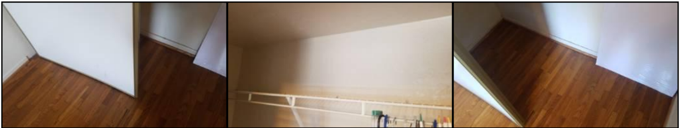
Bypass door guides missing at base - needs to be serviced
