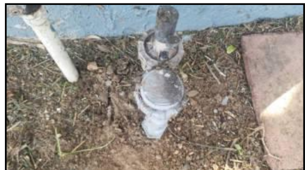
Stations not operating - needs to be serviced
