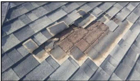
Deteriorated materials present - will require replacement at any time - consult a roofer to estimate remaining lifespan
