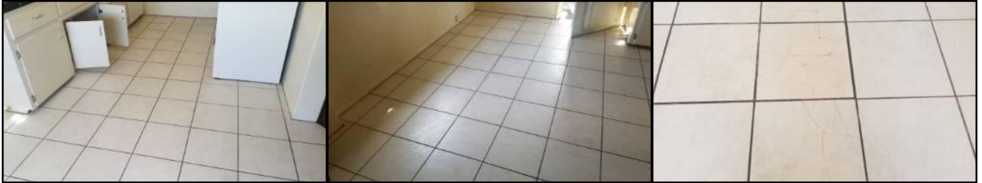
Cracked areas - needs to be serviced
