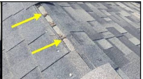
Missing/damaged shingles/tiles in areas - needs to be serviced
