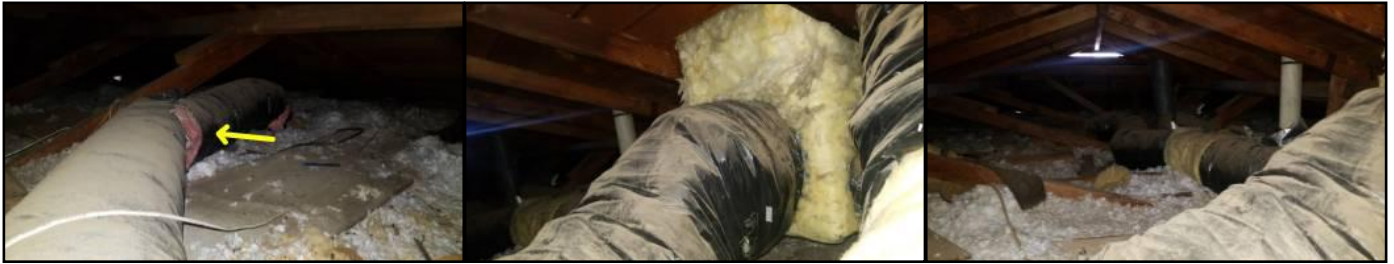
Outer wrap damaged - needs to be serviced
