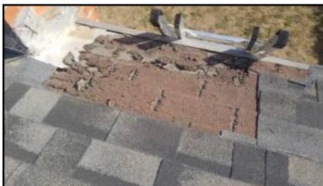
Deteriorated materials present - will require replacement at any time - consult a roofer to estimate remaining lifespan
