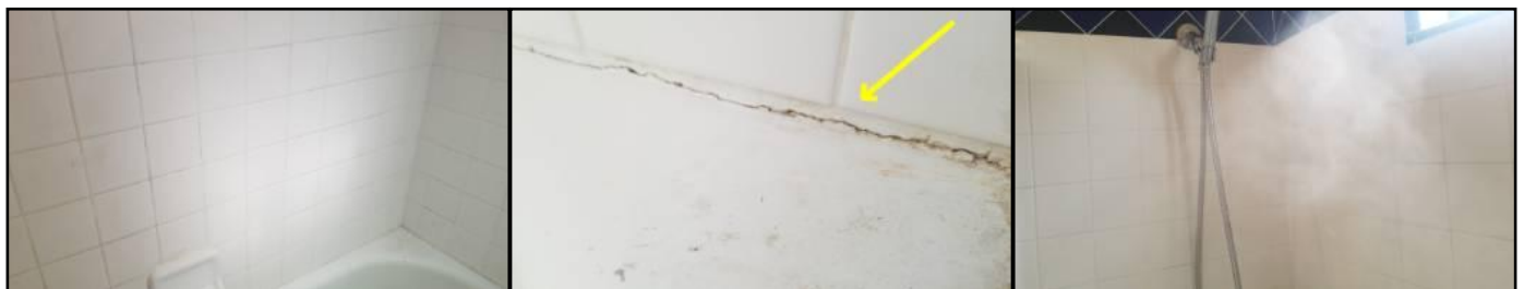
Worn tile/grout - typical for age - recommend routine grout and sealer maintenance
