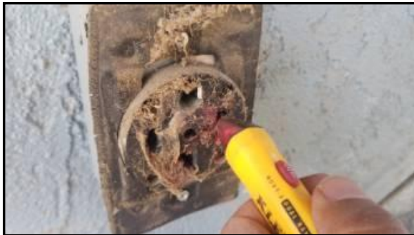
Has 240v service - tested and operated
