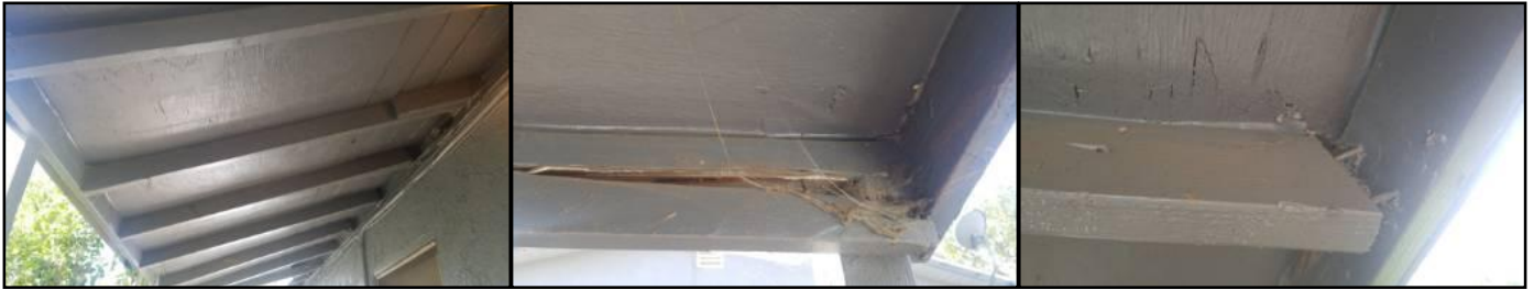
Wood deterioration observed - consult termite report
