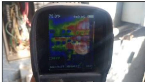
Thermal Image View - slight differential detected - monitor for further signs of overheating
