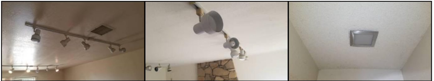
Some bulbs defective/missing/light(s) did not function - check bulbs/consult electrician to further evaluate
