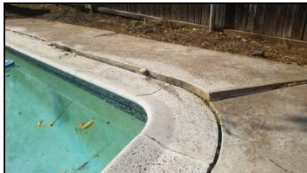
Uneven/lifted/lipage in areas – trip hazards present
