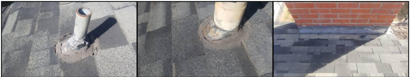
No saddle at high side of chimney - needs to be serviced
