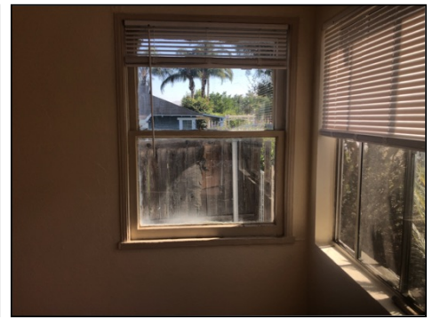
Stuck in position - needs to be serviced
