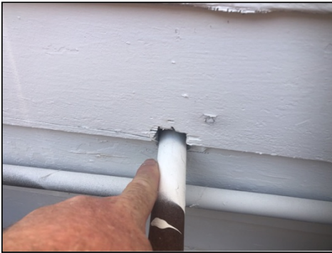
Small cracking/chipping/holes present - recommend siding service/maintenance and sealing all holes and gaps
