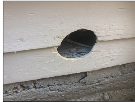
Cracking/chipping/holes more than typical - needs to be serviced
