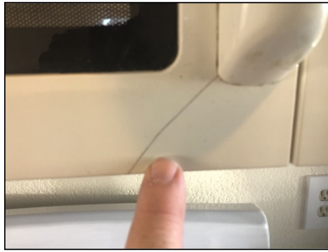
Visible cracks in door/frame - needs to be serviced
