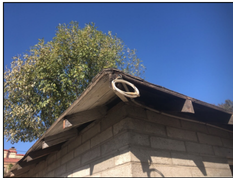
Exposed wires/connections - potential hazard - needs to be serviced
