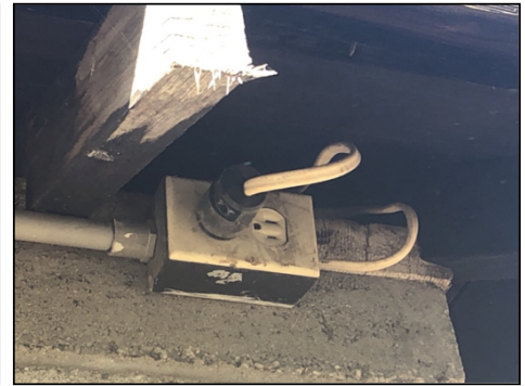
Exterior outlet/switch covers are missing or not of proper exterior weather proof type - needs to be serviced
