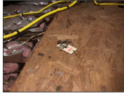
Evidence of rodent/bird/pest activity in the attic
