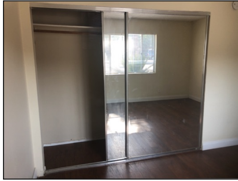
Bypass doors difficult to operate - needs to be serviced
