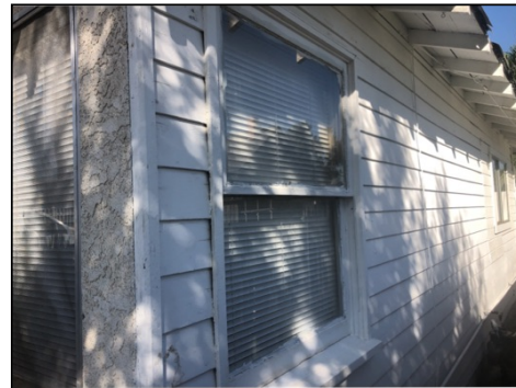
Worn windows/screens - typical for age
