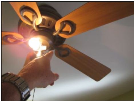
Pull cord missing at fan - needs to be serviced - north
