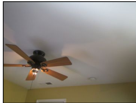
Missing light fixture globe - north
