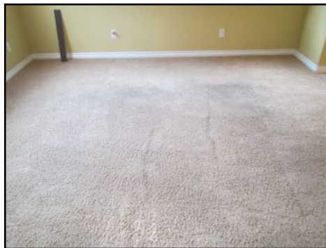
Loose carpet, recommend maintenance to prevent further loosening
