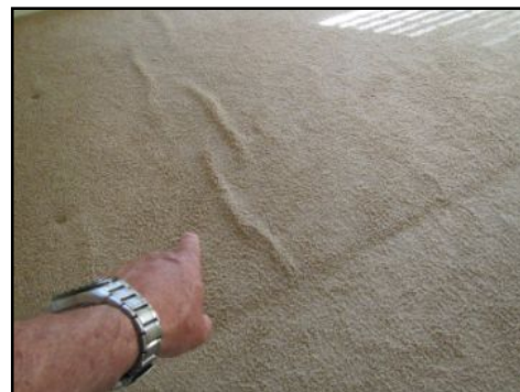
Loose carpet, recommend maintenance to prevent further loosening
