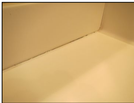
Gap at backsplash to countertop joint - needs to be serviced- master
