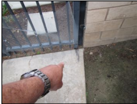
Gate rubs at side/bottom - needs to be serviced
