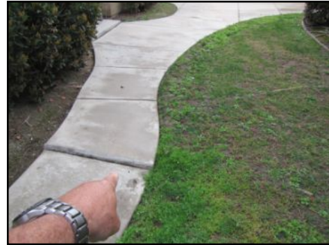
Tree/roots affecting walkways in areas - needs to be serviced
