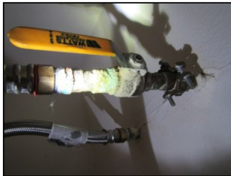
Corrosion at flexible connectors - needs to be serviced
