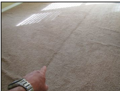
uneven floor - appears to be thicker/raised padding in part of the floor - master, recommend further evaluation
