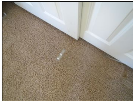
Bypass door guide broken at base - needs to be serviced - north
