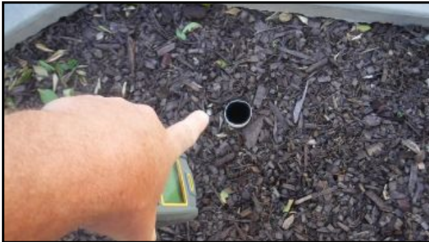
Unfinished drain installation present in areas of back yard. Poor drainage/standing water may occur in areas. Recommend evaluation/service.
