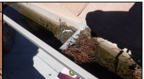
Gutters at south side of structure are clogged and not functional. Standing water present. Needs to be serviced.
