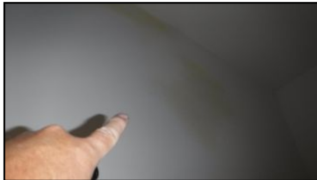
Patched/partial painted areas in closet present - southeast
