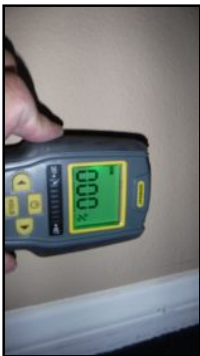
Wall areas adjacent to exterior planters of concern tested negative for active moisture.
