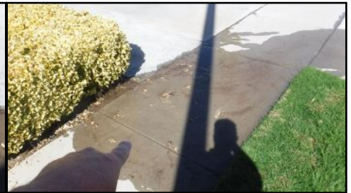
Underground leak/broken piping at southeast (by driveway)
