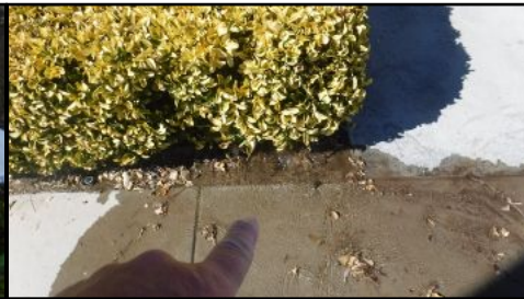
Underground leak/broken piping at southeast (by driveway)
