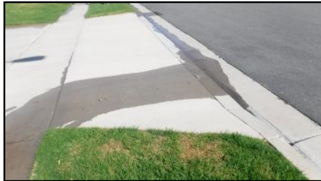
Underground leak/broken piping at southeast (by driveway)
