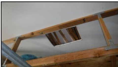
Hole present (ceiling) - needs to be serviced to retain integrity of fire separation
