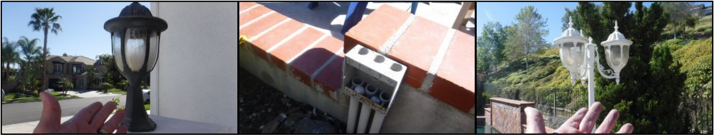
Unused/empty junction box at west side
