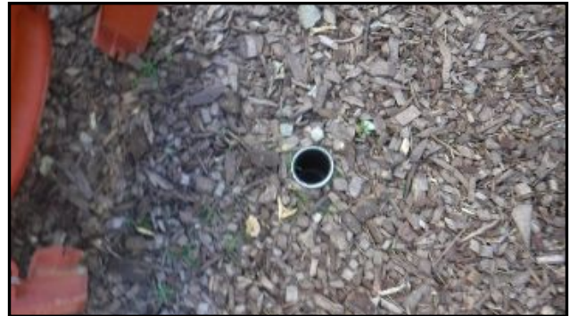
Unfinished drain installation present in areas of back yard. Poor drainage/standing water may occur in areas. Recommend evaluation/service.
