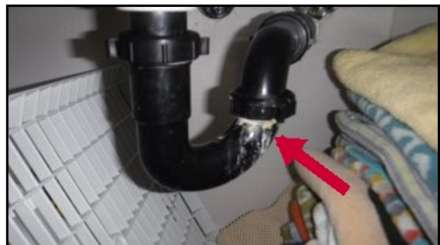
Dry corrosion at drain trap. Recommend evaluation.
