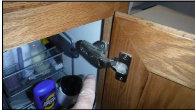
Loose hardware/hinge - southeast hall
