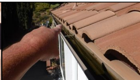
Gutters at south side of structure are clogged and not functional. Standing water present. Needs to be serviced.
