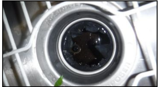
Unit corroded inside and at exterior casing. Visible leaking when unit is turned on. Replacement is recommended.
