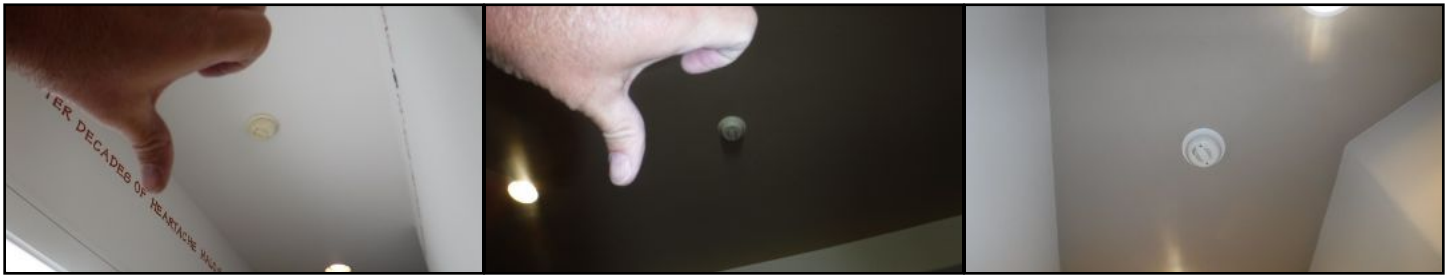
Did not operate near front entrance and at north hall - needs to be serviced or replaced
