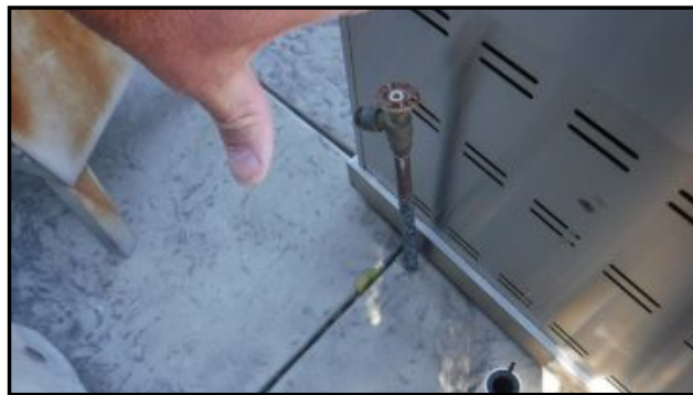
Faucet in back yard by bbq did not operate.
