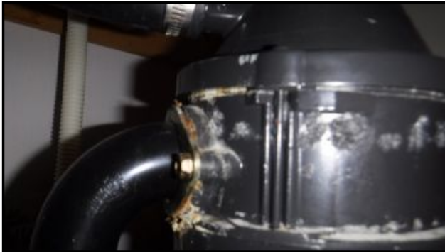
Unit corroded inside and at exterior casing. Visible leaking when unit is turned on. Replacement is recommended.
