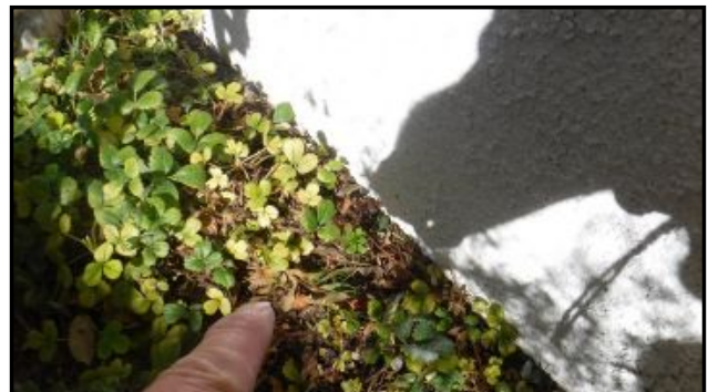
Soil in contact with weep screed in areas.
