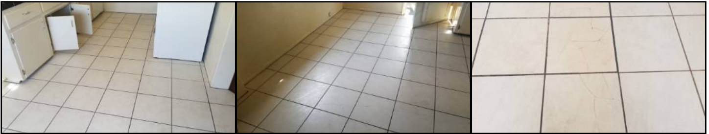
Cracked areas - needs to be serviced
