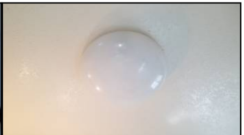
Some bulbs defective/missing/light(s) did not function - check bulbs/consult electrician to further evaluate
