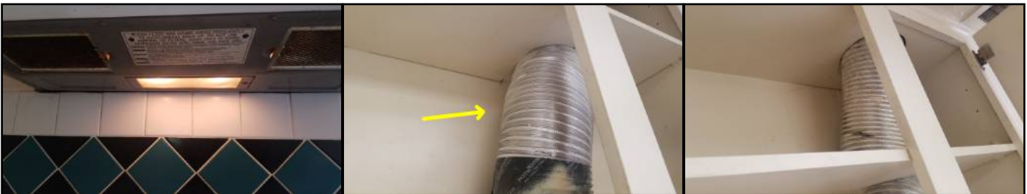
Improper vent materials used (ribbed flexible) must be smooth metal pipe - needs to be serviced
