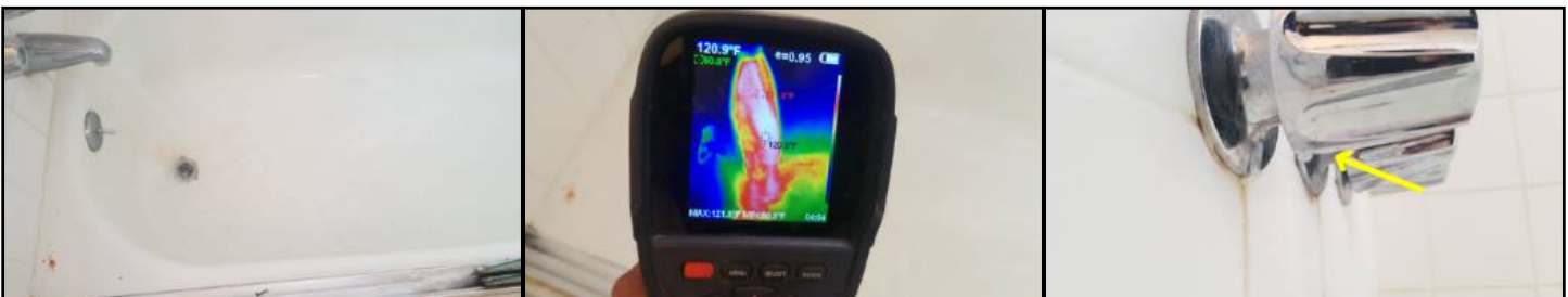
Tub fixture leaks when operated - needs to be serviced
