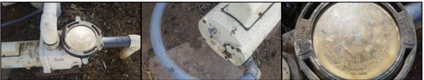
Missing bonding wire
