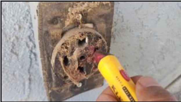
Has 240v service - tested and operated
