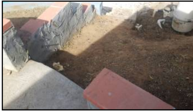
Missing steps - unsafe - needs to be serviced
