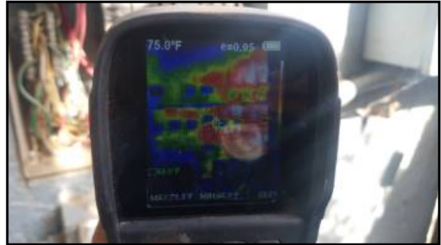
Thermal Image View - slight differential detected - monitor for further signs of overheating
