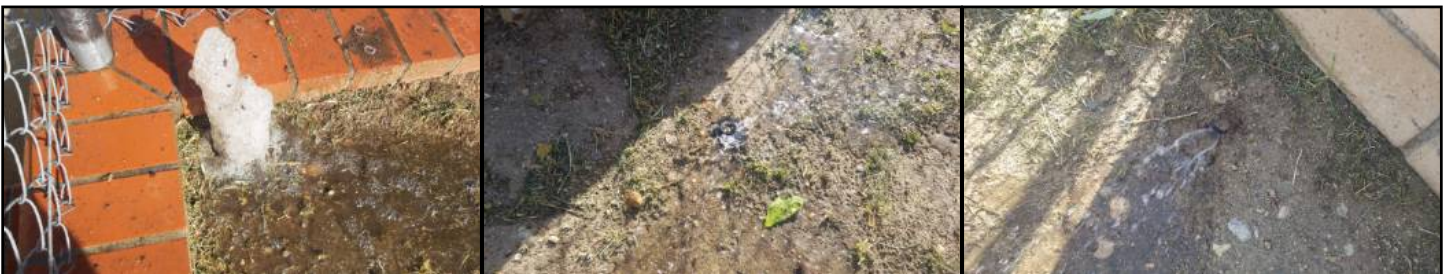
Missing sprinkler heads - needs to be serviced
