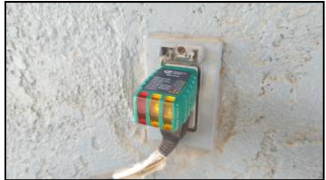
Missing exterior cover
