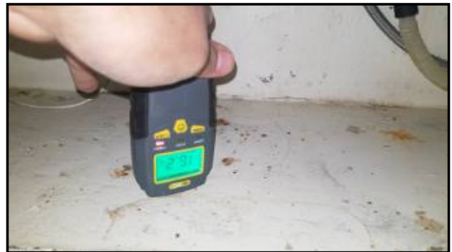
Stained/blistered area(s) - moisture present at time of inspection - needs to be serviced/further evaluated
