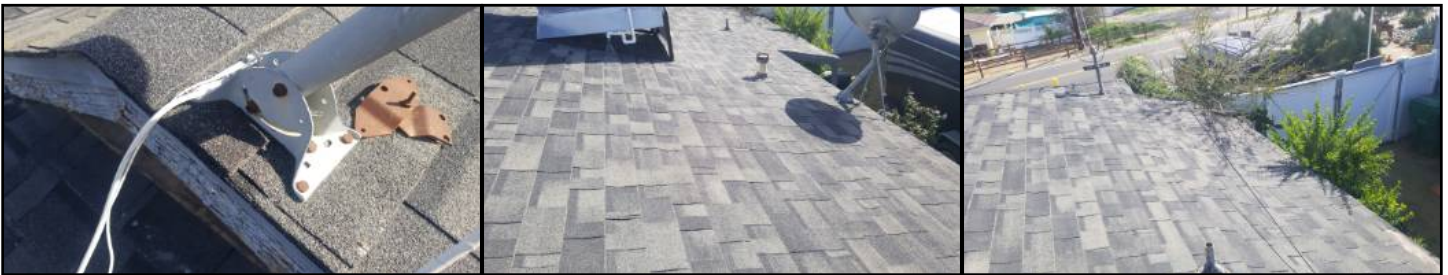
Satellite dish fastened direct to roof - screws will need periodic caulk maintenance
