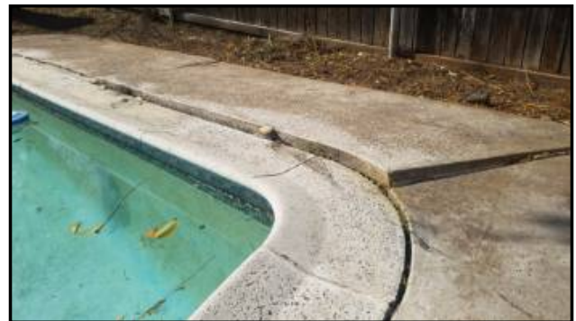
Uneven/lifted/lipage in areas – trip hazards present
