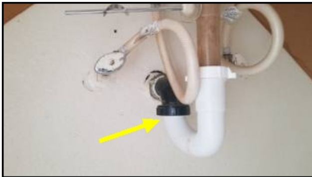
Visible leaking under sink - needs to be serviced
