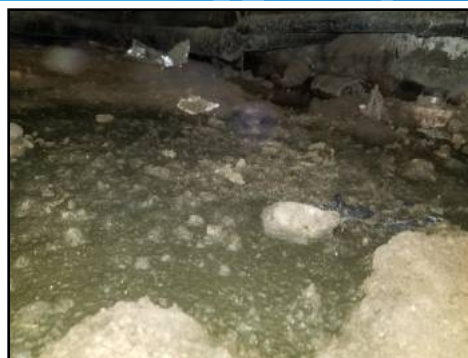
ground is extremity damp in areas
