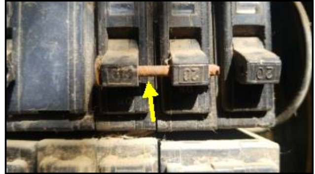
Improper breaker tie
