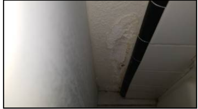
Damaged in areas - needs to be serviced
