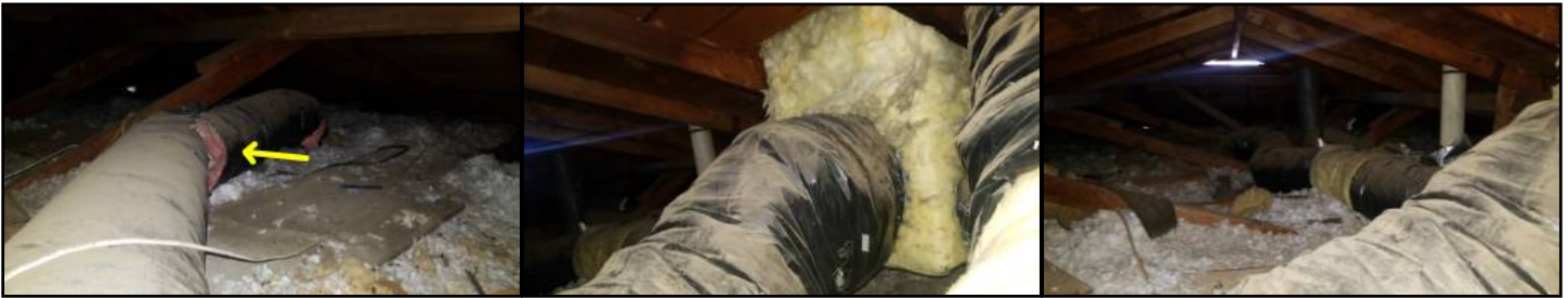
Outer wrap damaged - needs to be serviced
