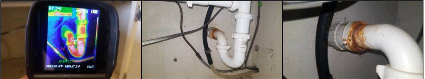
Corrosion is present at plumbing areas - this is a sign of slow leaking and should be serviced
