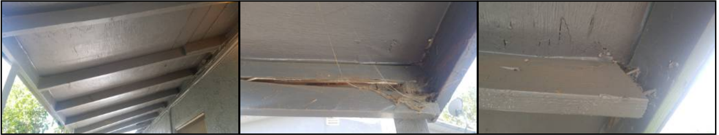
Wood deterioration observed - consult termite report
