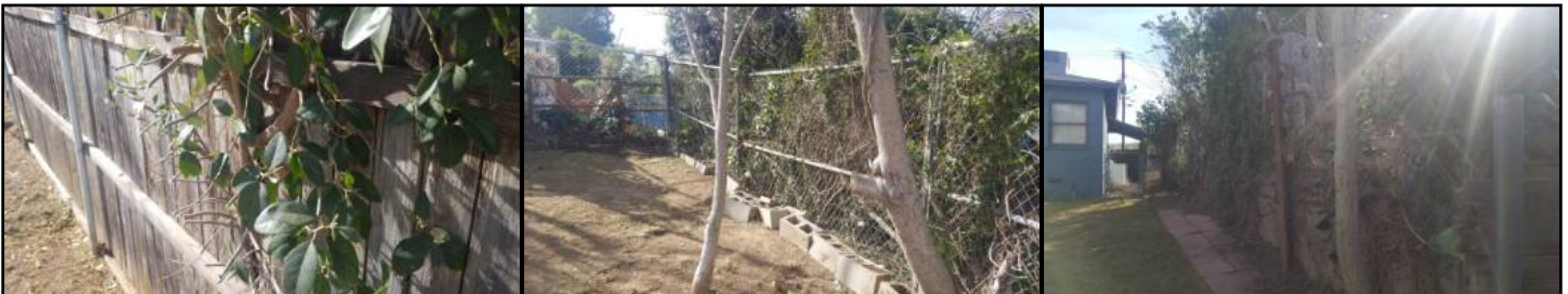
Vegetation or trees are affecting the fencing/walls in areas - needs to be serviced
