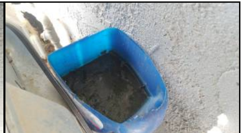
Drain trap is clogged - needs to be serviced
