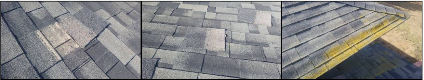
Missing/damaged shingles/tiles in areas - needs to be serviced
