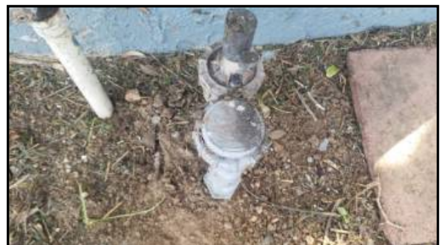
Stations not operating - needs to be serviced
