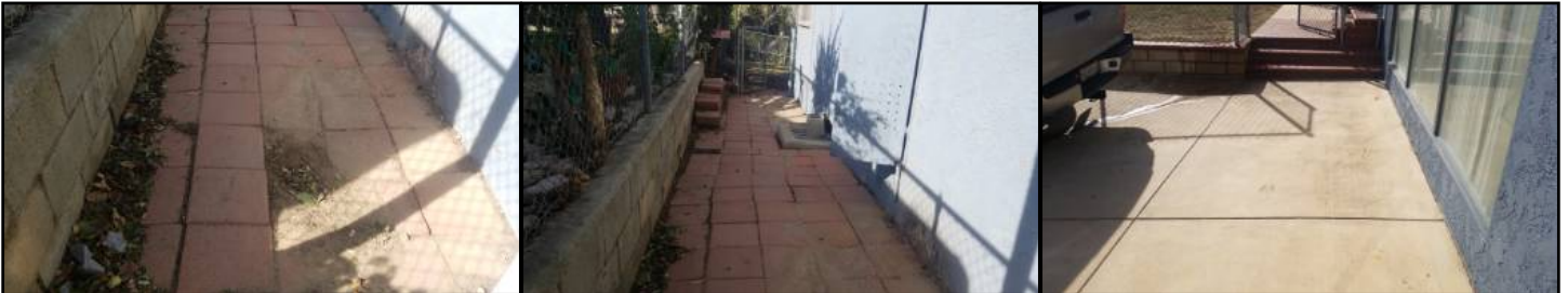
Walkway displacement/uplifted/uneven areas - potential trip hazard - needs to be serviced
