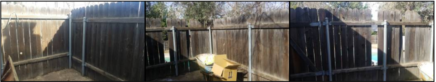
Damaged fencing/walls - needs to be serviced
