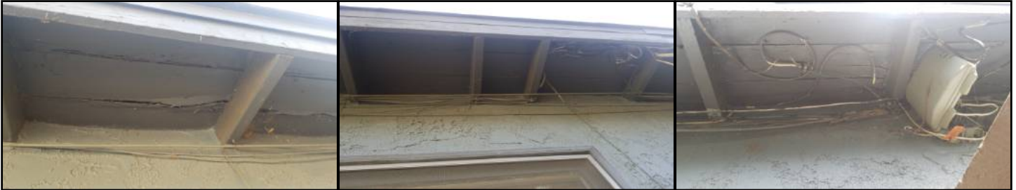
Deteriorated in areas - needs to be serviced - consult the termite report
