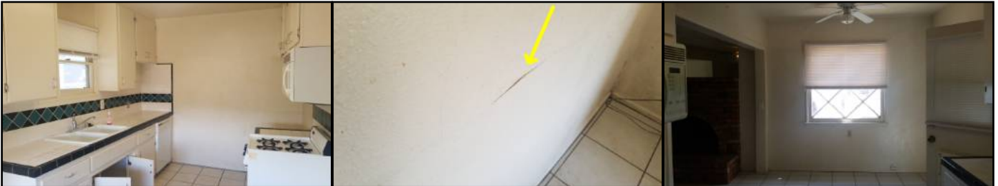
Large crack - recommend servicing
