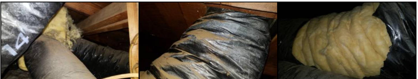
Outer wrap damaged - needs to be serviced
