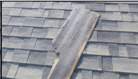
Missing/damaged shingles/tiles in areas - needs to be serviced
