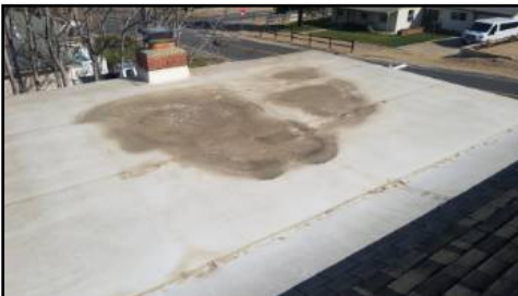
Ponding or evidence of ponding in areas - needs to be serviced
