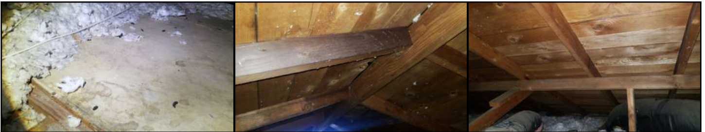
Evidence of rodents/pests - recommend pest services inspection for further evaluation
