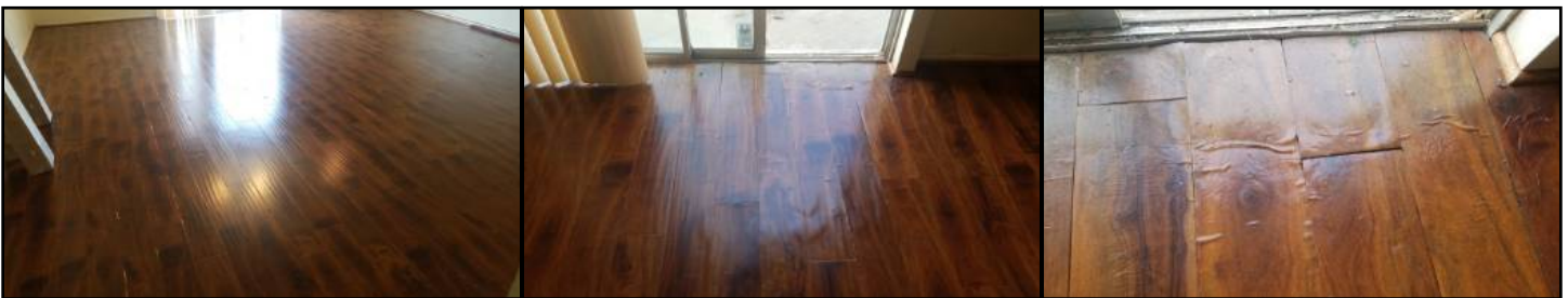
Wood flooring is swollen/cupping/lifting - evidence of a past moisture problem - needs to be serviced
