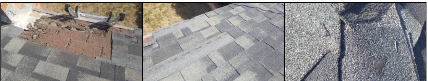
Deteriorated materials present - will require replacement at any time - consult a roofer to estimate remaining lifespan
